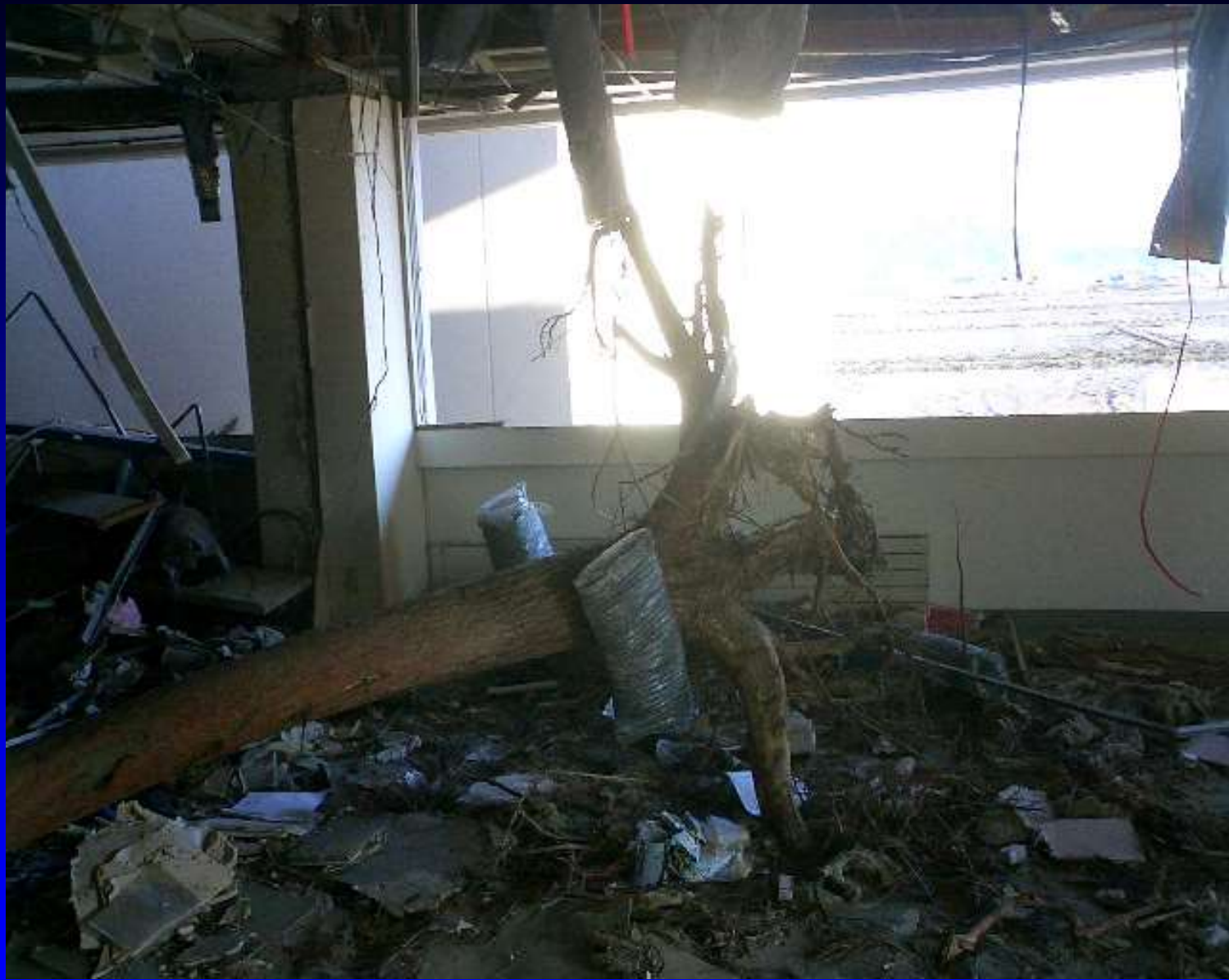
Interior of damaged hospital, Iwate Pref, Jan. 2012, Photo by Leo Bosner
